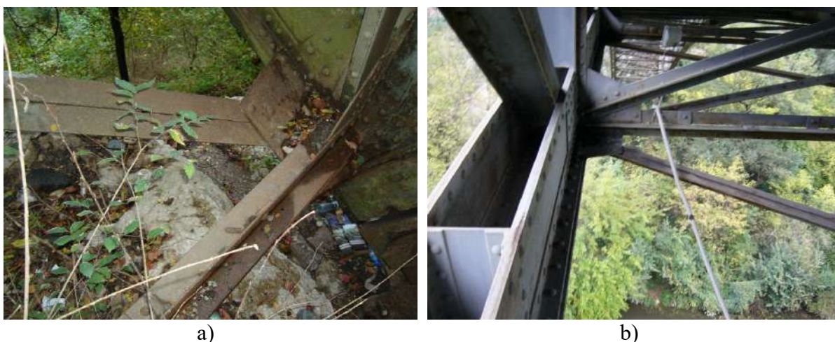
Figure 4. Corrosion of the bridge structure: a) the contact with the masonry foundation, 2009 (photo by Mandev, Partov) b) detail of the arched lower chord, 2009 (photo by Mandev, Partov)
