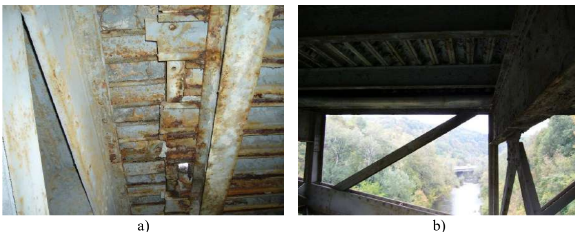
Figure 3. Corrosion of the bridge structure: a) detailed of the track structure from below, 2009 (photo by Mandev, Partov) b) detail of the horizontal beams, 2009 (photo by Mandev, Partov)
