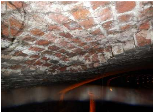
Figure 6. Pushed out brickwork layer
